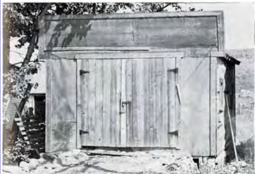
OLD SINGLE GARAGE USED FOR EQUIPMENT STORAGE. A HAZARD TO EQUIPMENT AND THE COMMUNITY
